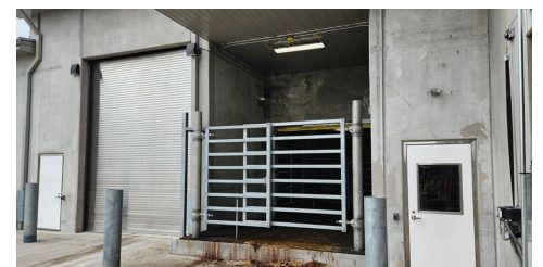
Delivering with a gooseneck trailer? We have you covered! Take a look at this loading dock.
