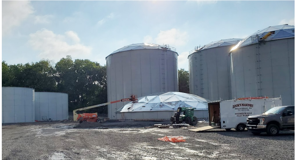
Five tanks have been erected at the Nicholas Meat Sustainable Resource Facility (SRF) and the remaining six tanks for the project's first phase will be erected by the end of the year.
