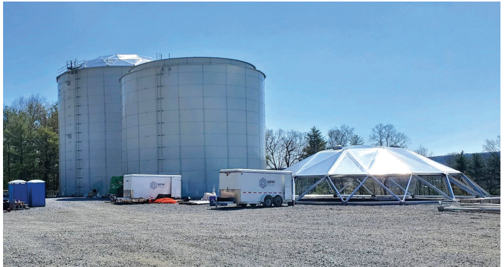
Tanks at the Sustainable Resource Facility will become more prominent as construction continues this summer.
