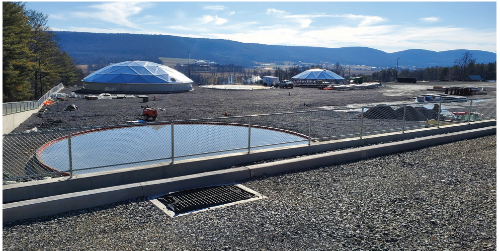
Tanks are beginning to take shape at the Sustainable Resource Facility. Shown here is the roof, or dome, of a tank as well as a section of wall material. As the tank is built, rings of the wall material will be added until the tank is at its full height.
