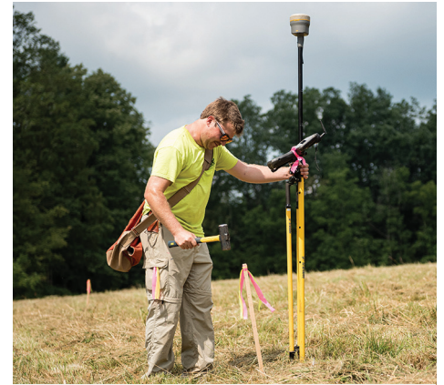
A worker marks an area at the Sustainable Resource Facility as work continues on the project.
